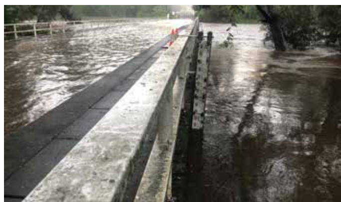
View of flooded Silverdale Road Bridge, Wallacia, March 2021 flood. Source: Wallacia Rural Fire Brigade
